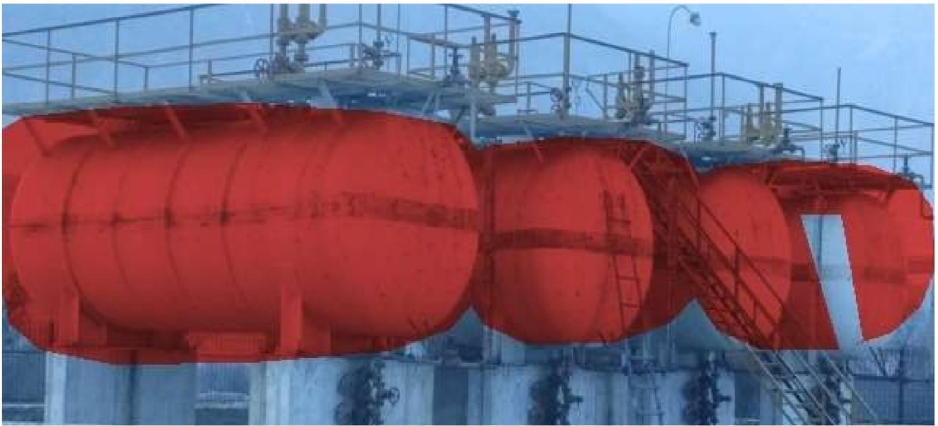
LPG Storage & Filling Facility – Representative Site View
