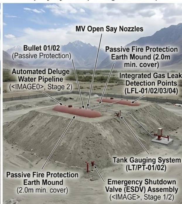
Figure D: Completed Mounded Storage Bullets & Passive Fire Control
