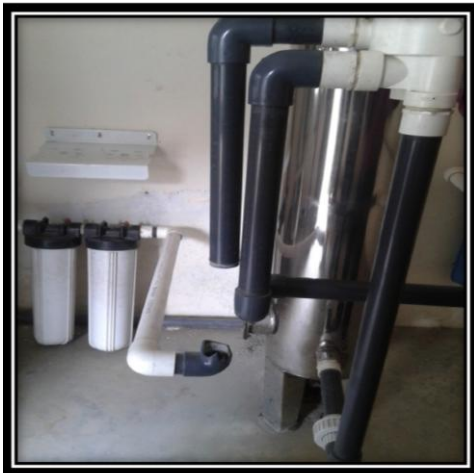
Fig. 3. Broken pipeline at Old polo ground WPP, Gilgit.
